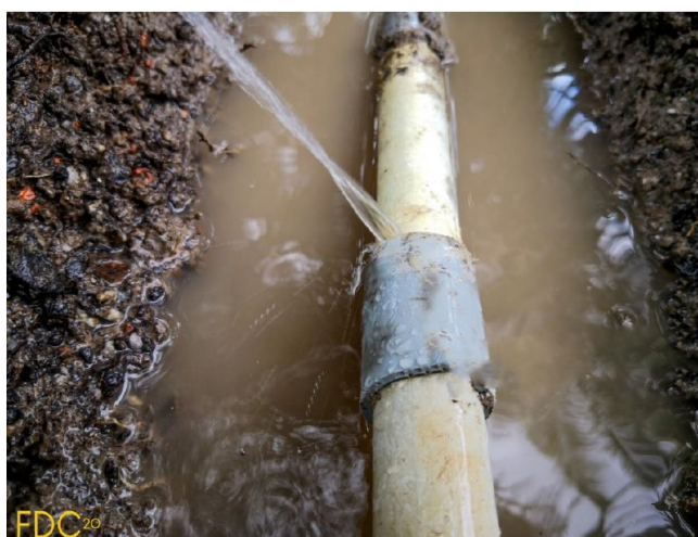
Figure 21, lack of management and maintenance leaves the condition of the individual pipelines to the respective users' responsibility (Chikuhwa, 2021)
