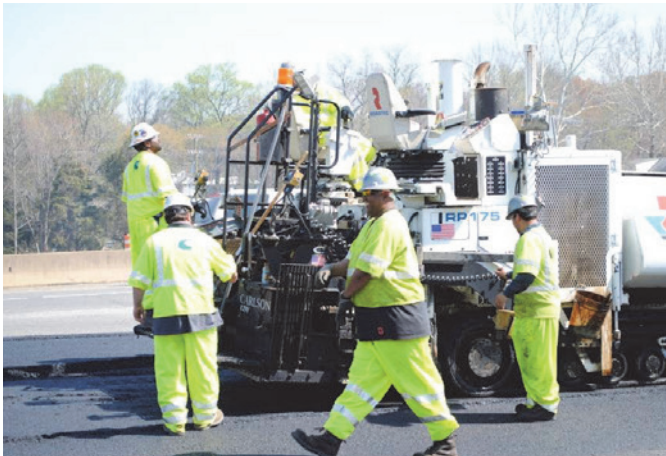
FIGURE 21 – ALL WORKERS WEAR SIMILAR HIGH-VISIBLE CLOTHES (PHOTO COURTESY OF THE AMERICAN ROAD & TRANSPORTATION BUILDERS ASSOCIATION.)
