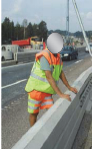
FIGURE 18 – EXAMPLE OF GOOD HIGH-VISIBILITY WARNING CLOTHING (SUMMER)
