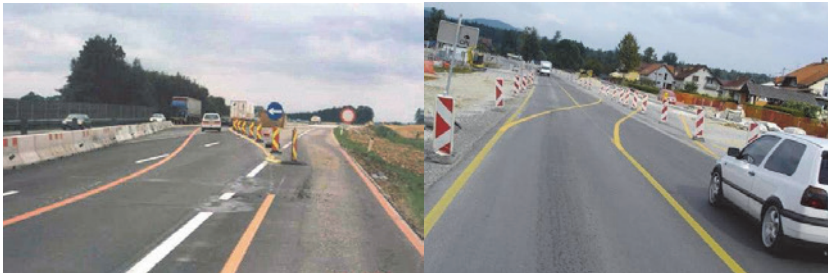
FIGURE 12 – CORRECT (OLD MARKINGS GONE) INCORRECT (OLD MARKINGS STILL VISIBLE)
