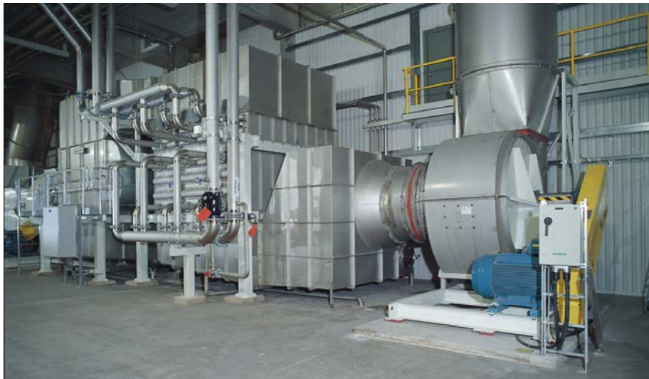
Figure 4.1. Heat Recovery Tower.
