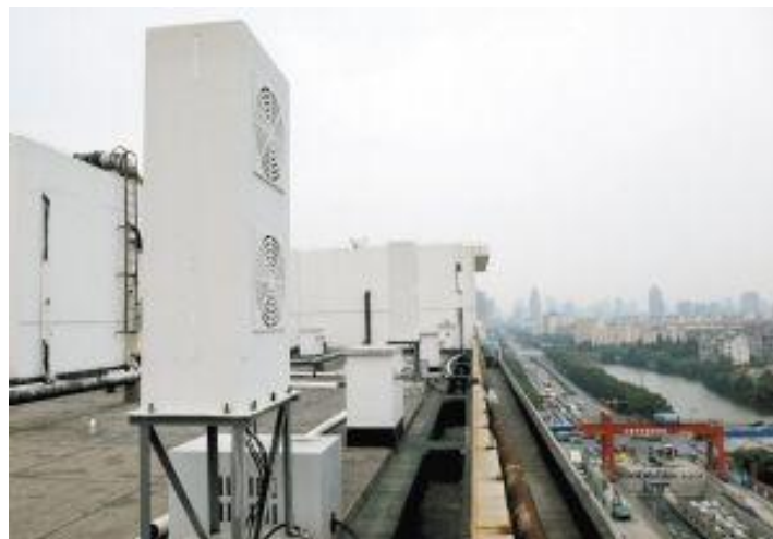
Figure 3.4-4: Air conditioner external unit-like site. [21ic]
