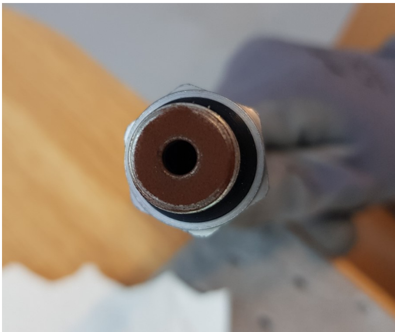
Figure 21. Dust deposit on buffer tank A inlet from CRU.
