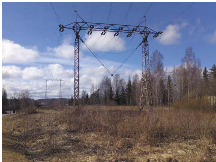
Figure 1. Rautarouva, 110 kV line in Riihimäki. Photograph: Heinäaro, Kimmo
