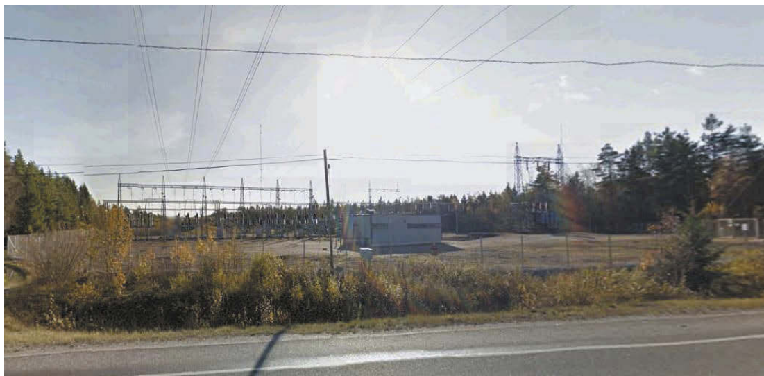
Figure 8. Photograph of a power substation. Screenshot: Google Streetview
