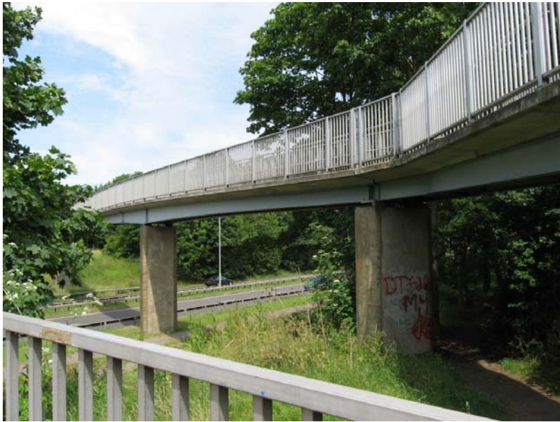
31. Stevenage, Hertfordshire, June 2006: "graffiti is sprayed all over the concrete bridge supports".
