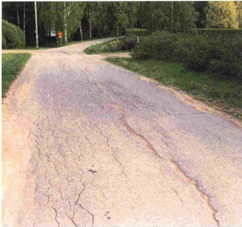
Figure 8: Rajalantie in Luopioinen, Finland – before renovation
