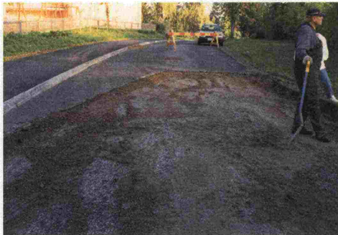
Figure 12: Fiber-ash section opened for control
