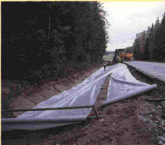
Protecting groundwater against salt and other chemicals in Pernaja in 1994 (Main Road 7).
