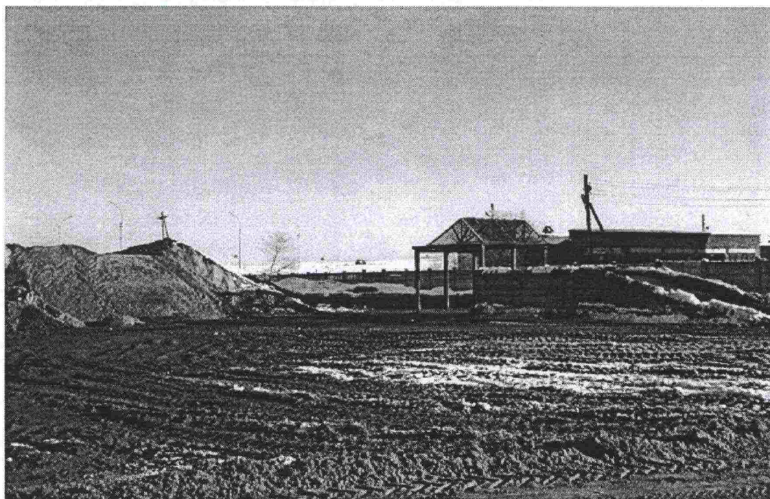
Figure 3. Road maintenance areas still store salt-sand and salt outside. This causes the material to cake, making it difficult to use. The ramp in the photo facilitates loading, although it could have been made even more functional.
