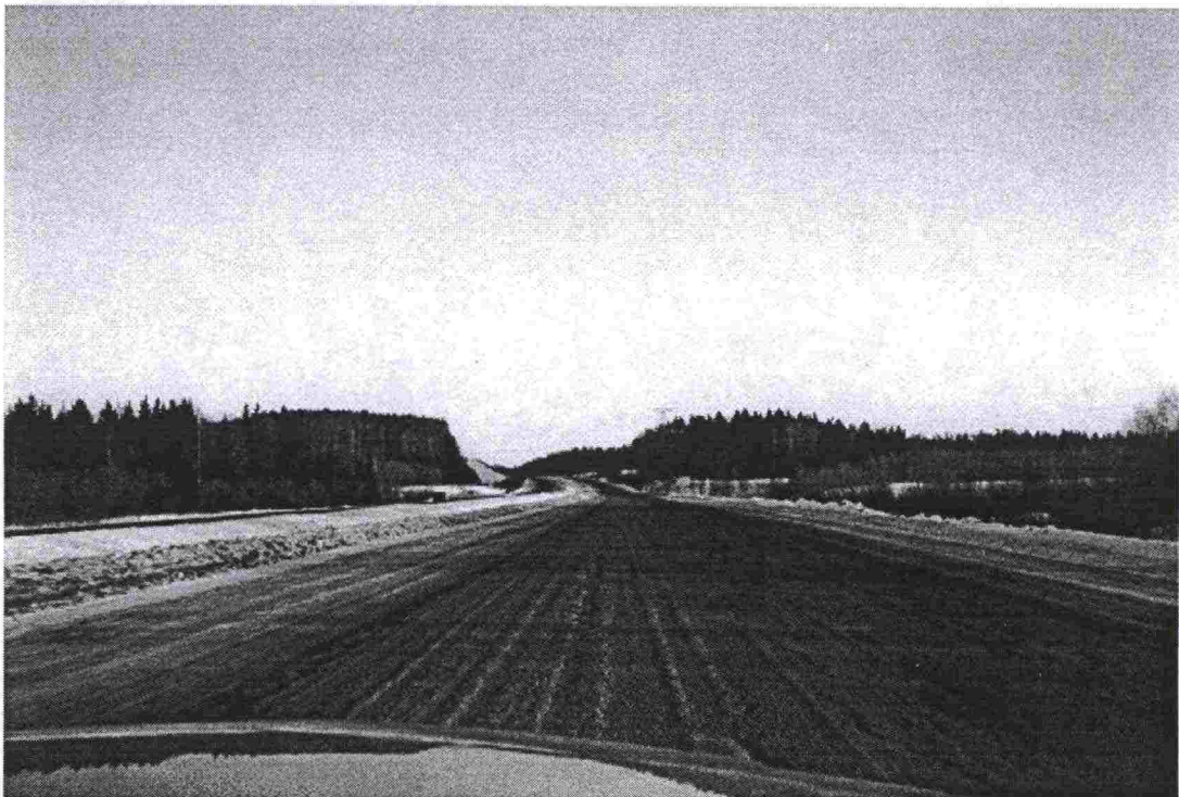
Figure 2. Some roads have deteriorated rapidly due to pavement failure.
