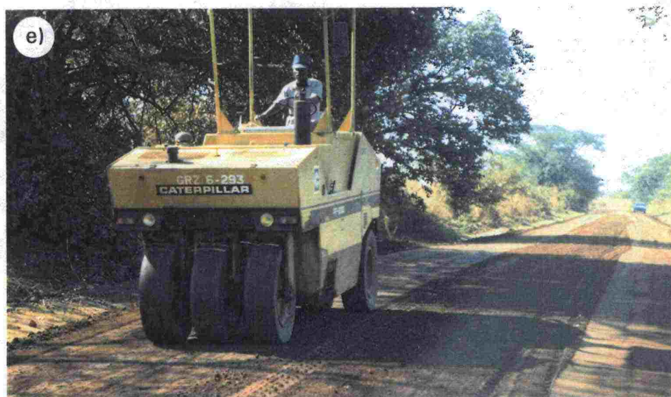
Figure 30. Stabilization work on district road D177 near Lusaka in Zambia in June 1991. d) Mixing and/or grading with a grader, e) Compaction with a pneumatic roller. (See the previous Figure!)
