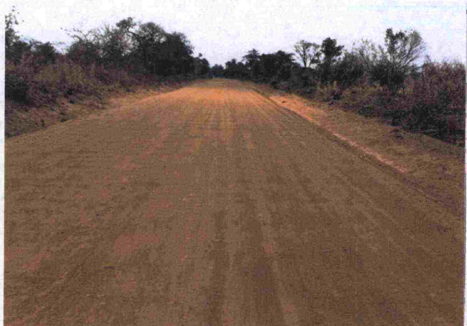
Figure. Class 2. The shape of the road may have changed. There are many corrugations, ruts or potholes and most of the surface is not solid. Very dusty.
